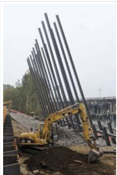
Piles along the Columbia River at the Port of Vancouver are being installed to support a trench allowing trains to pass under a bridge spanning the river. The work is part of the port’s 10-year, $275 million West Vancouver Freight Access project. (Photo by Sam Tenney/DJC)
