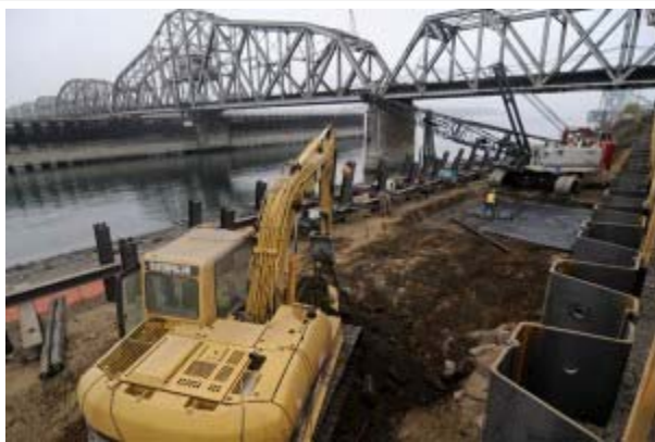
Crews with Hamilton Construction build a trench at the Port of Vancouver that will ease rail congestion by allowing trains entering the port to pass under the Columbia River Rail Bridge. (Photo by Sam Tenney/DJC)
