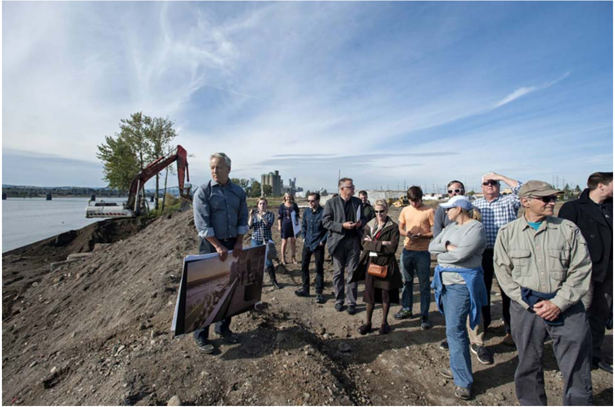
Developer Barry Cain, left, checks out the view while leading a tour Tuesday afternoon of the Vancouver Waterfront construction site. (Photos by Amanda Cowan/The Columbian)
